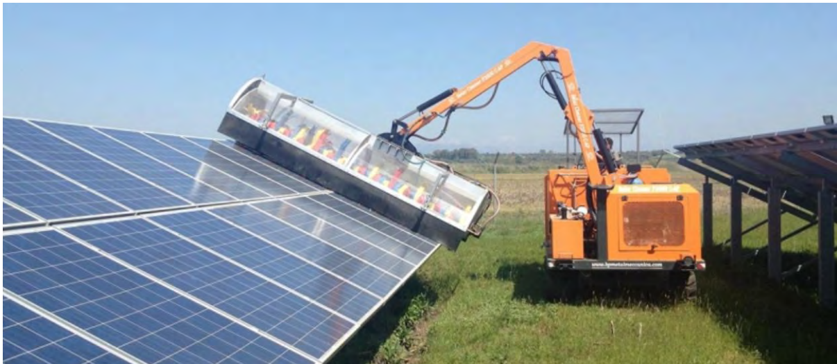
Figure 14 – Solar farm cleaning equipment
